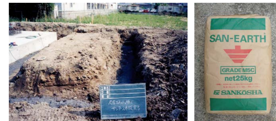
Laying SAN-EARTH M5C *One 25kg bag of M5C will cover approx. 3 meters (width 50cm).
